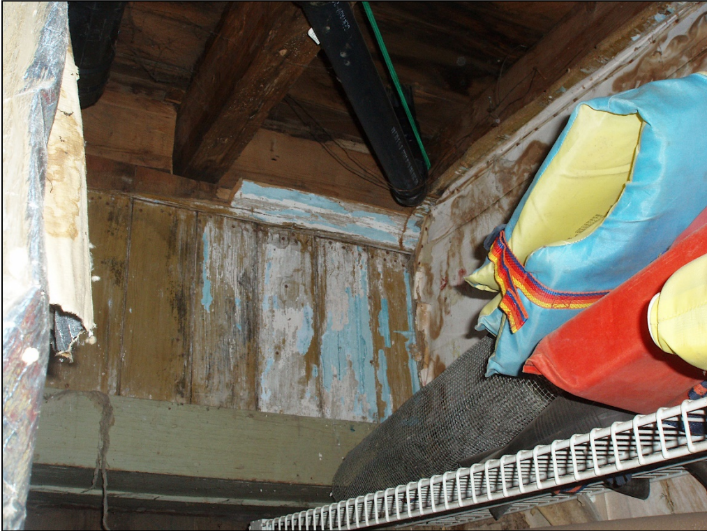
Photo 18 of 19: Webber Lake Hotel Prussian Blue Paint in Room 104
